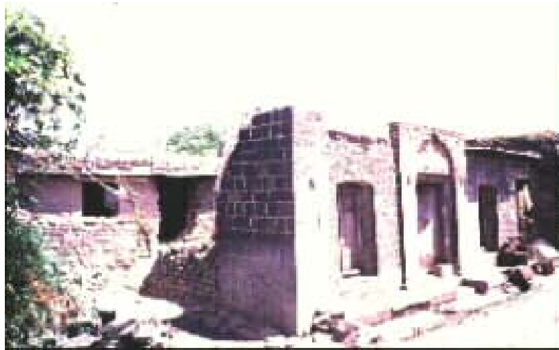
Fig. 7.6 Behind nice traditional façade, the housing fabric has deteriorated considerably
