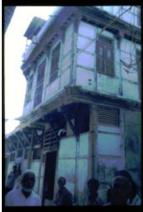
Fig. 8.9 Traditional house with projecting floor joists supported by struts in timber located in Limbdi. These performed well during 2001 earthquake
