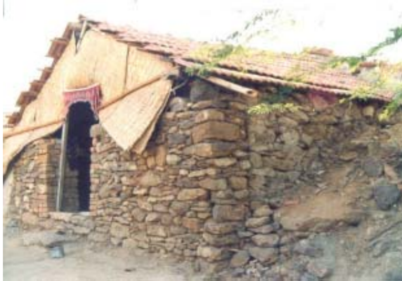
Fig. 8.23 Changes made to the semi-permanent structure by raising the walls making it unsafe. Sep. 2001
