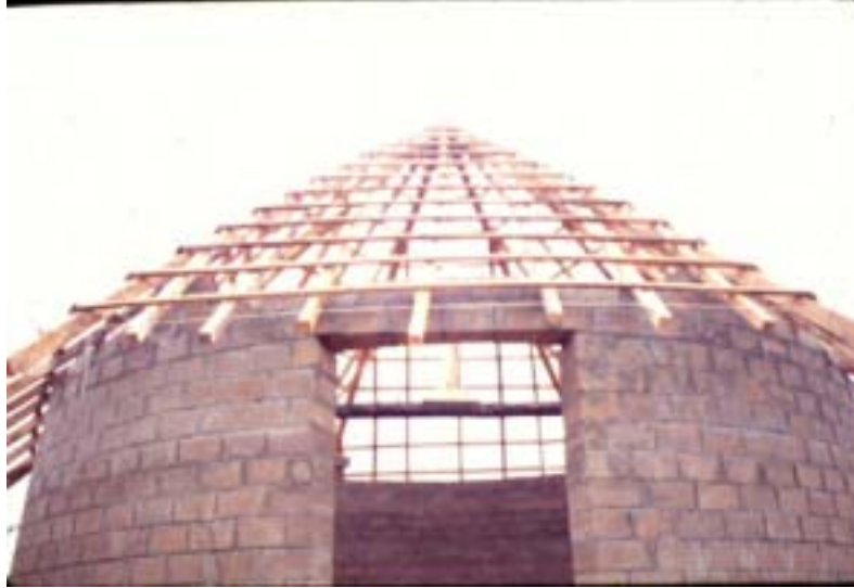
Fig. 8.25 Modern traditional Bhungas in compressed soil blocks, ring reinforcement and wooden rafters, promoted by Abhiyan Sep. 2001
