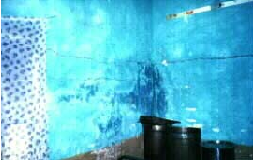
Fig. 7.18 Cracks in reconstructed houses due to earthquake in June 2000
