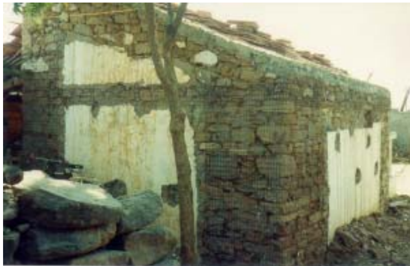
Fig. 8.27 Retrofitting of a vernacular construction in village Makhna through application of wiremesh for corner strengthening Oct. 2001
