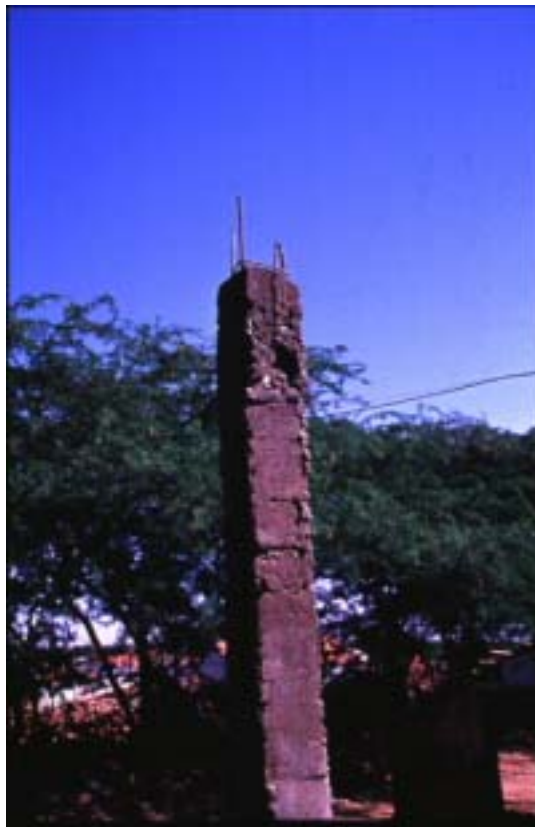
Fig. 8.33 The column in the new construction is of very poor quality- village Nani Cherai Oct. 2001
