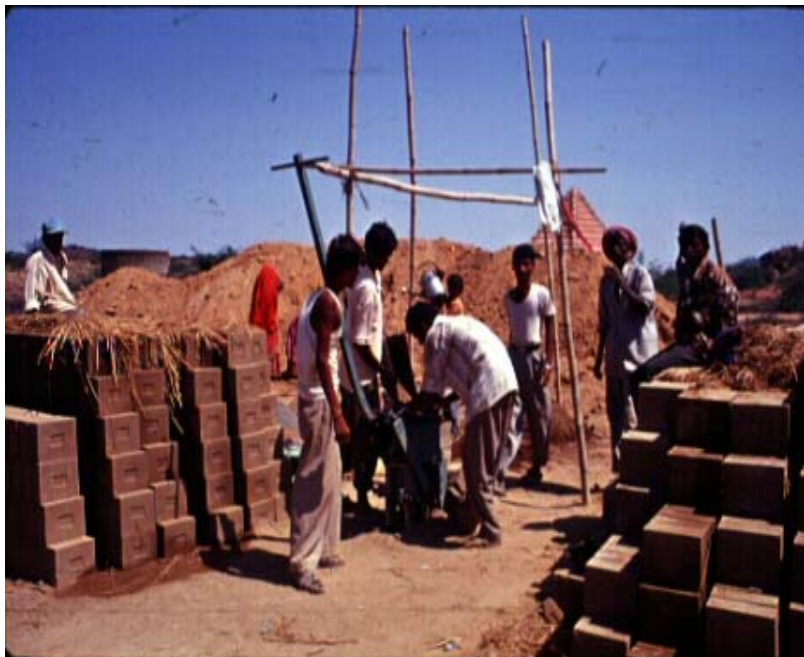
Fig. 8.32 The use of compressed soil blocks advocated by Abhiyan by mixing 90-95% soil and 5-10% cement, dried in shade for 3 days and then cured for 20 days Oct. 2001
