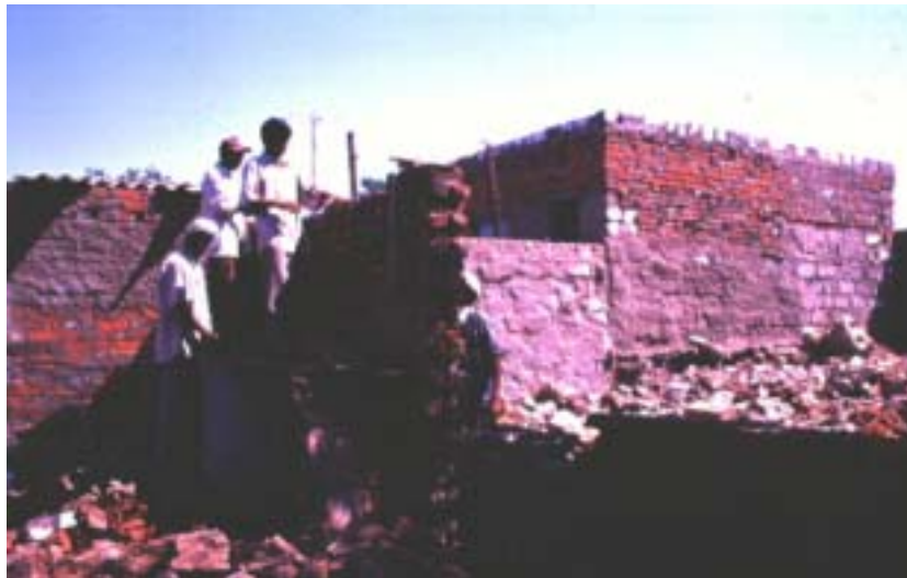
Fig. 8.18 Poor self help constructions in Bhachao using variety of materials. Sep. 2001
