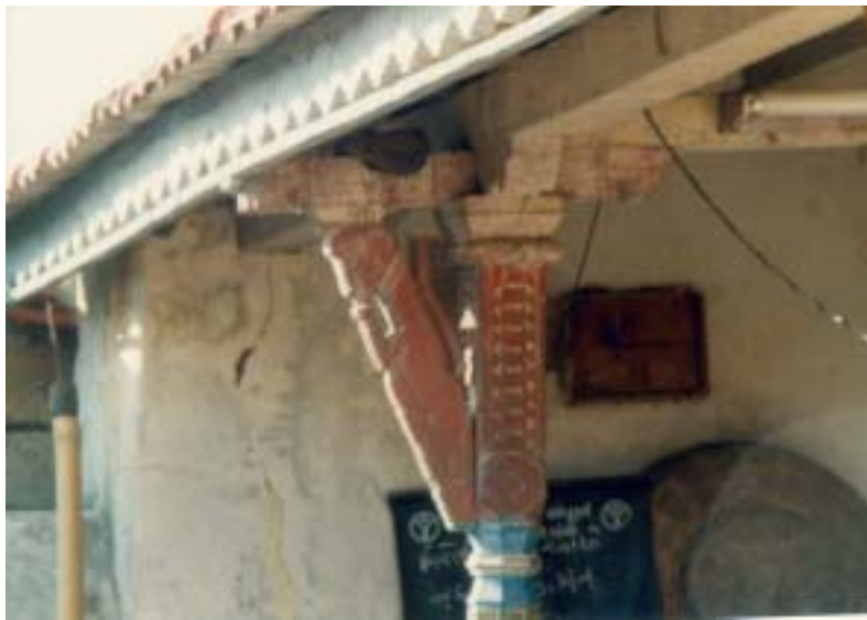
Fig. 8.10 & 8.11 Tie beams and knee bracing in traditional housing of Kutch are very effective in resisting lateral forces of earthquakes.
