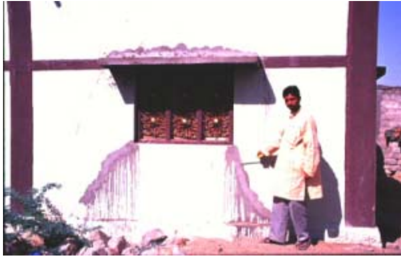
Fig. 8.34 The cracks, no matter how deep they are, are just filled with cement grout Oct. 2001
