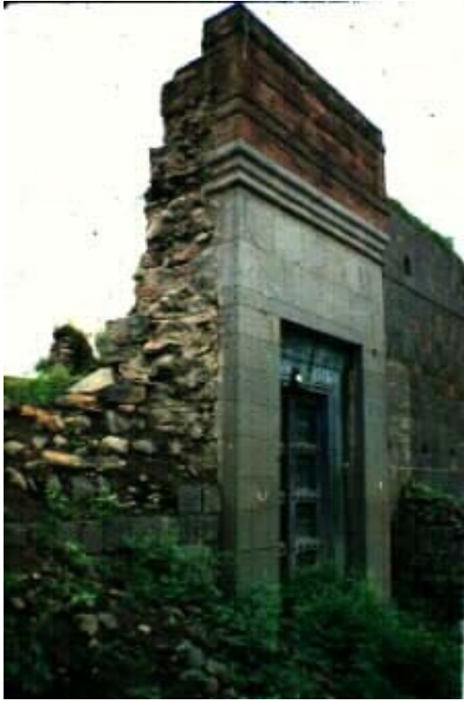
Fig. 7.8 Traditional walls with random rubble masonry in mud mortar are poorly bonded
