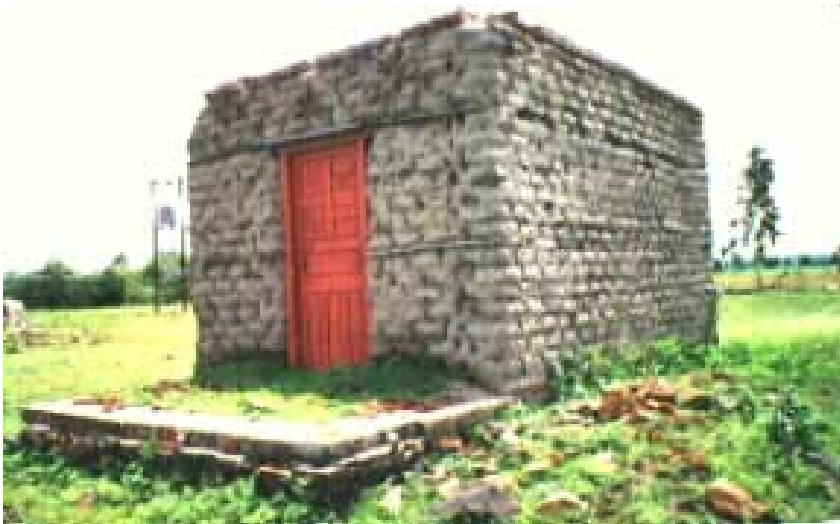
Fig. 7.20 Model house to demonstrate seismic resistant adobe construction lying in ruins
