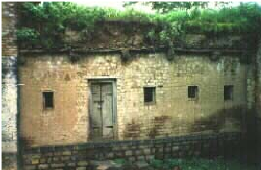
Fig. 7.7 Heavy traditional roof due to accumulation of mud layers
