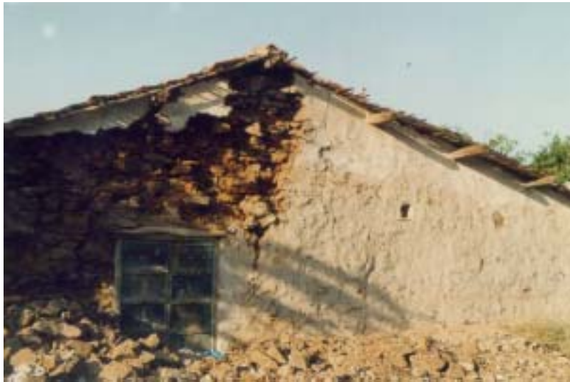
Fig. 8.13 Poor rubble masonry in vernacular constructions of Kutch prior to 2001 earthquake
