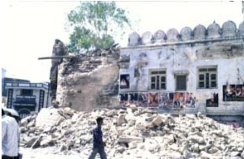
Fig. 8.15 The earthquake caused severe damage to various heritage components such as historic wall of Bhuj Feb. 2001
