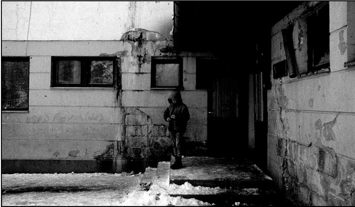
Fig.6.4.3 The settlement in the forest in Banovici. What was once thought of as a possible future post-war hotel is today a dilapidated structure, made almost uninhabitable by extreme neglect on the part of the tenants, lack of maintenance and unsound construction.
