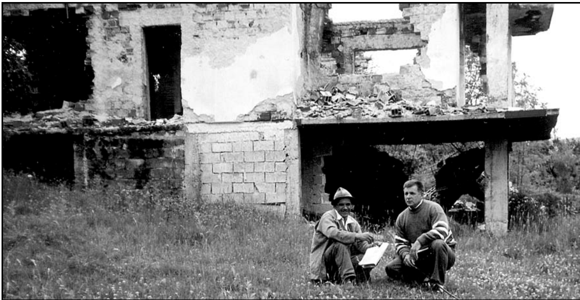
Fig. 6.5.13 a, b Four stages of reconstruction. This page: a) Ekrem Buljbasic in front of his house in Grapska in the summer of 1996; b) in front of the house 1997 with one of the Serb IDPs. The clay blocks of the external walls have now been smashed (continued on next page)
