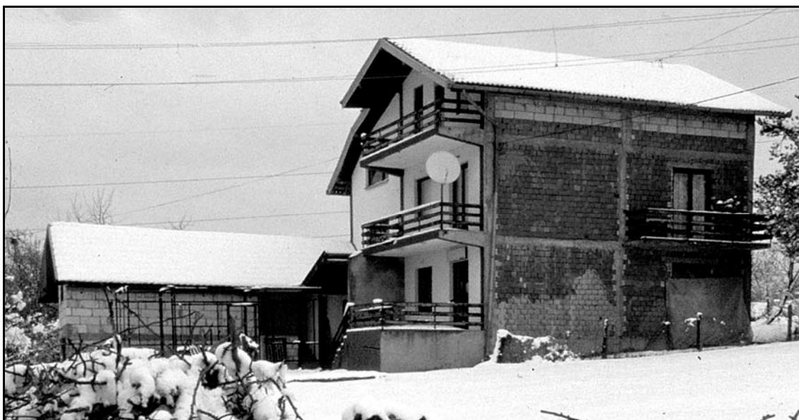
Fig. 6.3.5 The largest of the empty houses in Kiseljak Breze. 144 people were to live here. The owner stayed in Croatia throughout the war and never returned. The house is all but empty and due to lack of maintenance is showing signs of advanced dilapidation.
