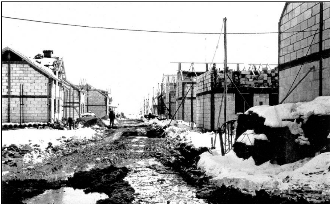
Fig.6.4.11 Constructing the 'Mihatovici houses' in Prutace in February 1996 revealing the seasonal difficulties in constructing floor slabs in timber. In Bosnia, even today, there is normally no 'exposed' construction going on in winter.
