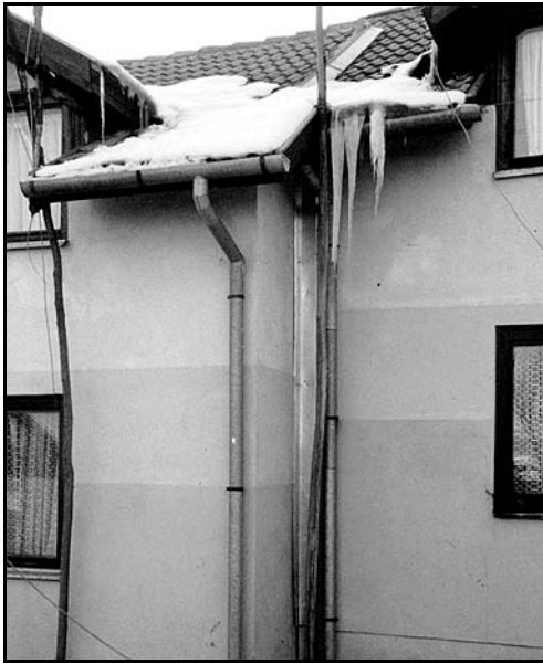
Fig.6.4.10 Detailing where two units of construction meet. The roof constructions were not correctly designed (or constructed) and caused endemic leakages. Note the flashing on the roof.
