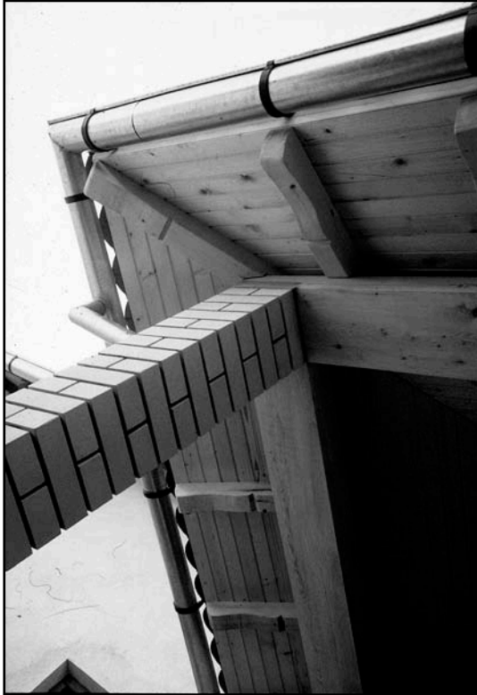
Fig. 6.5.21 The level of workmanship was excellent at least where professionals had been employed, like in this case where work of the mason, the carpenter and the tin smith bears little resemblance to 'but-it-was-war' quality referred to in my other two cases.
