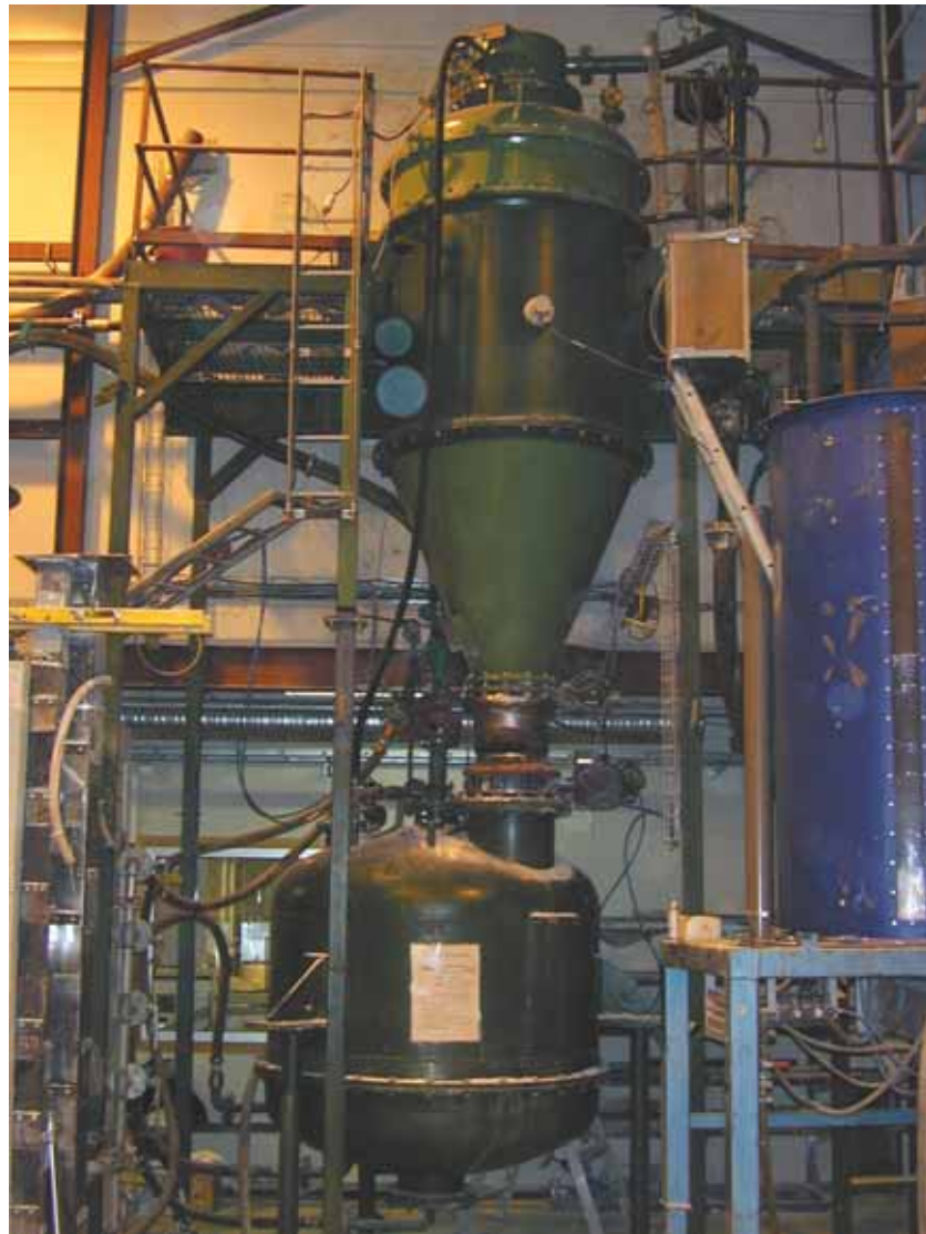
Figure 3-4: The blow tank and the receiving tank.
