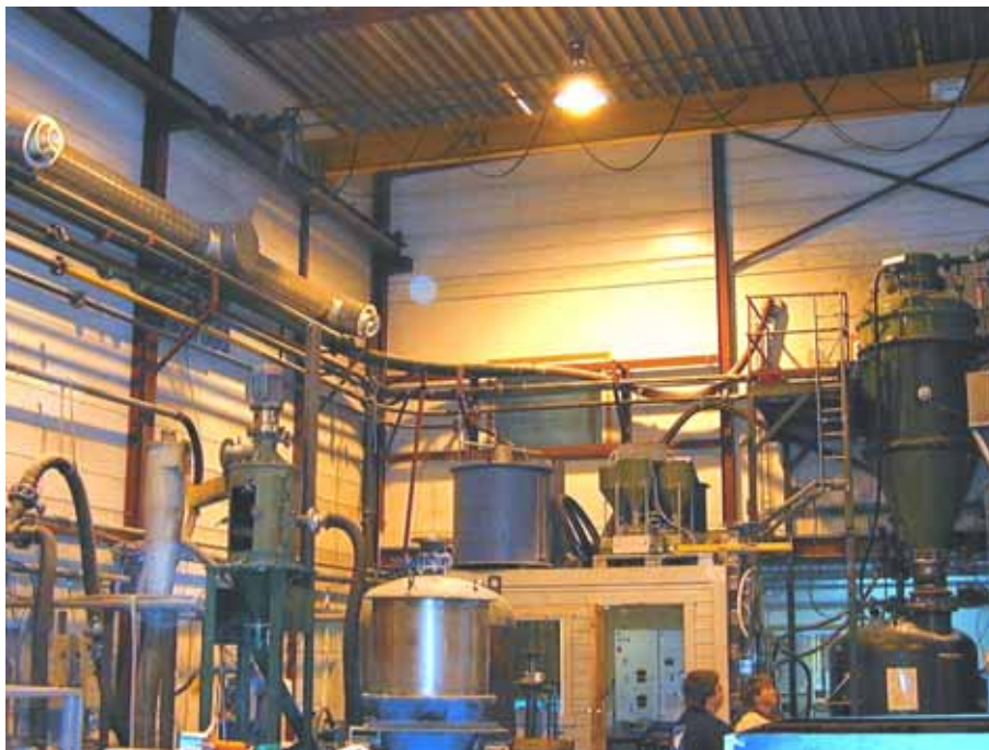
Figure 3-5: A part of the conveying pipeline.
