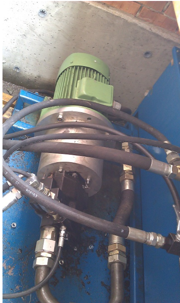
Figure 13: The hydraulics pump engine.
