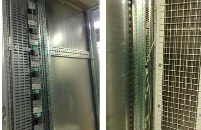
(a) A ladder for power (b) A ladder for data cables
