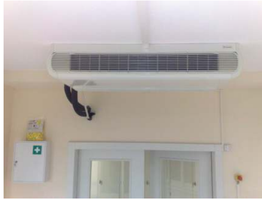
Figure 2.16: Daikin HVAC ready for use.
