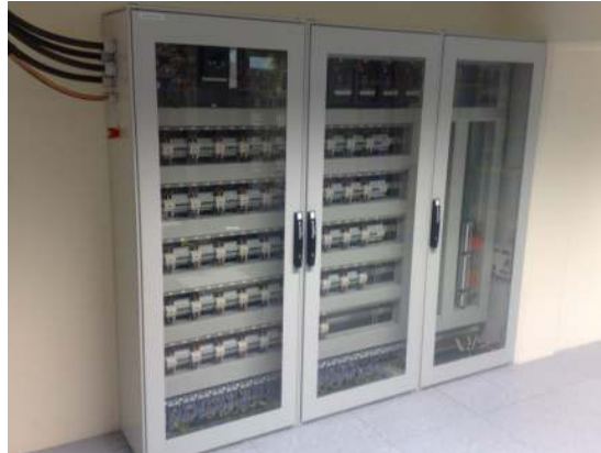
Figure 2.10: Distribution panel installed in the laboratory
