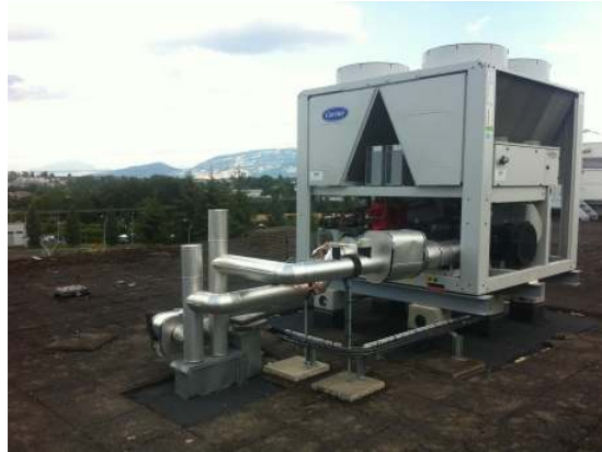
Figure 2.13: The 30RB Aquasnap chiller which is installed on-top of building 4
